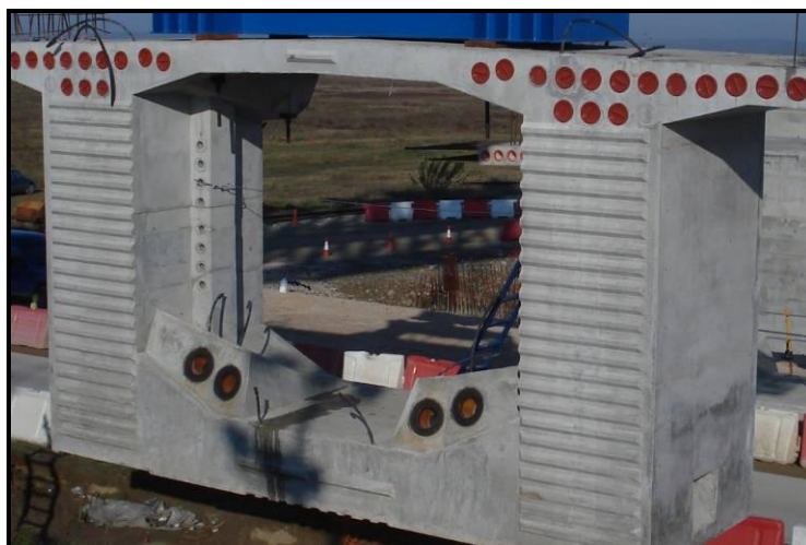
Fig. 8 Severe Radius of Tendon Exiting at Anchorage Blister
